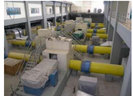
Fig 4. Pumping station Source: [Inc., 2019]
