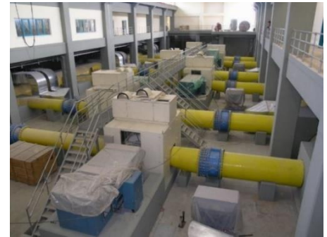
Fig 4. Pumping station Source: [Inc., 2019]
